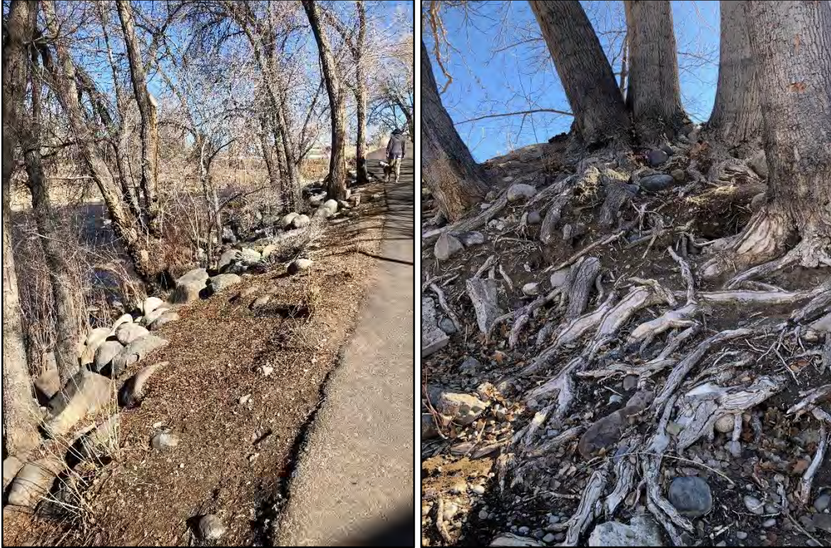
Figure 7. Rocked bank with trees near Kuenzli Bridge remain stable (photo left). Large trees and root systems hold the slope on the downstream end of project (photo right).
