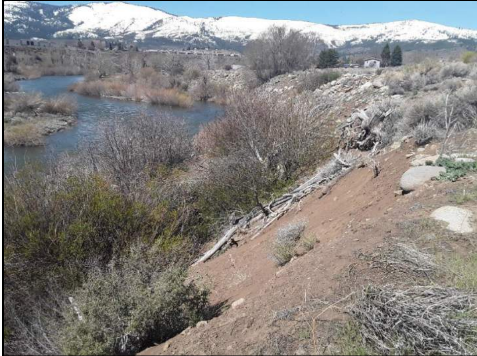
Photograph A-1. Verdi roundabout parcel. Washoe County, L13, L14. Steep river bank with high cover of debris on the slope (L14).
