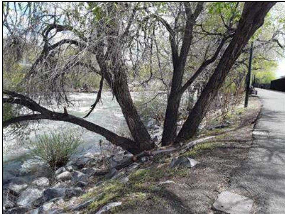
Photograph A-11. Sutro Street through John Champion Park. City of Reno, L73, L74, L75, L76, L77. Angular riprap is placed in many areas, however, erosion is still occurring on the steep slopes (L74).
